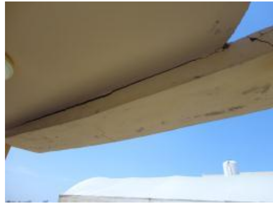
Poor quality – Cracks Sammouni area / Gaza city - April 2013
