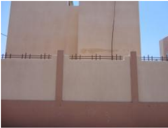
Poor quality – Leakage Khan Younis city - April 2013
