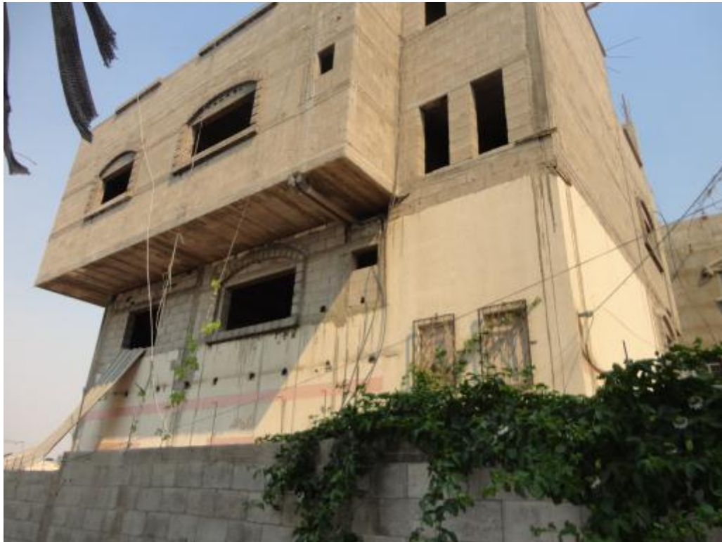
Adding another floor to the housing unit Sammouni area / Gaza city - April 2013
